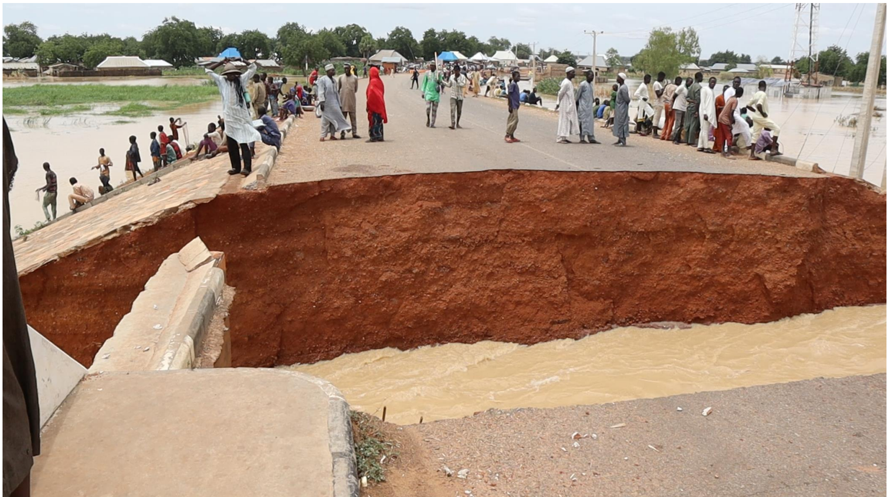
Bridge washed away by flood in kebbi state
